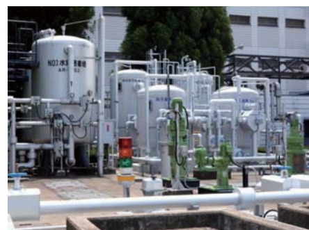
System for treating wastewater from research for reuse at the Central Research Laboratories
